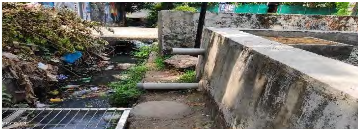
Figure 7.3: Discharge of Blackwater into Open Drains
