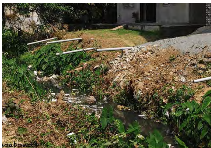
Figure 3.3: Wastewater (mostly grey) led out into nallahs
