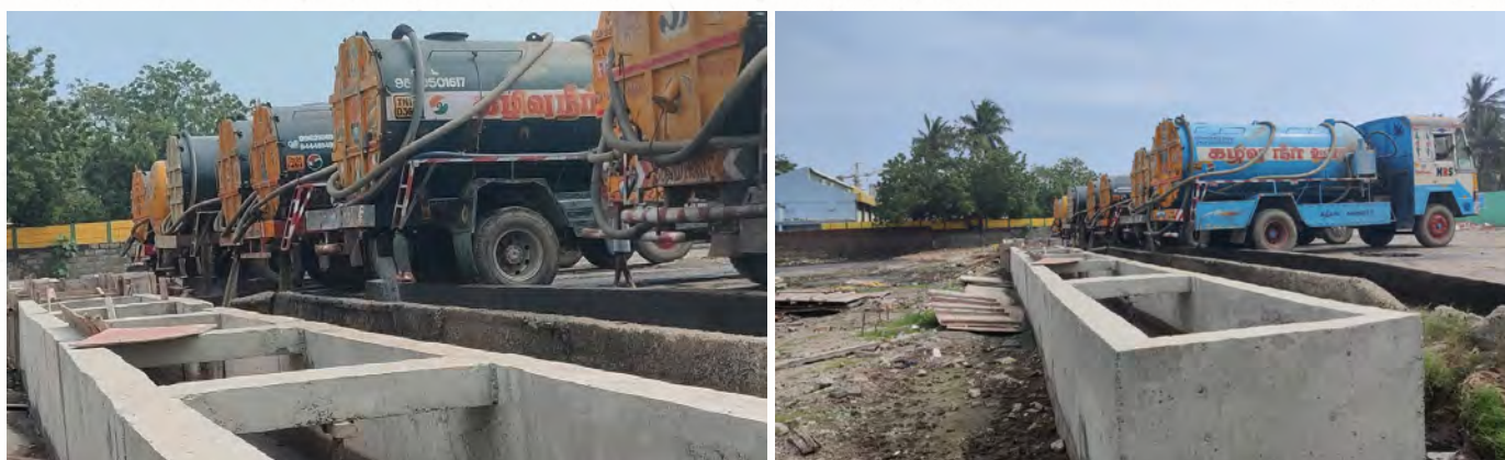
Figure 9.8: Decanting facility at the STPs
