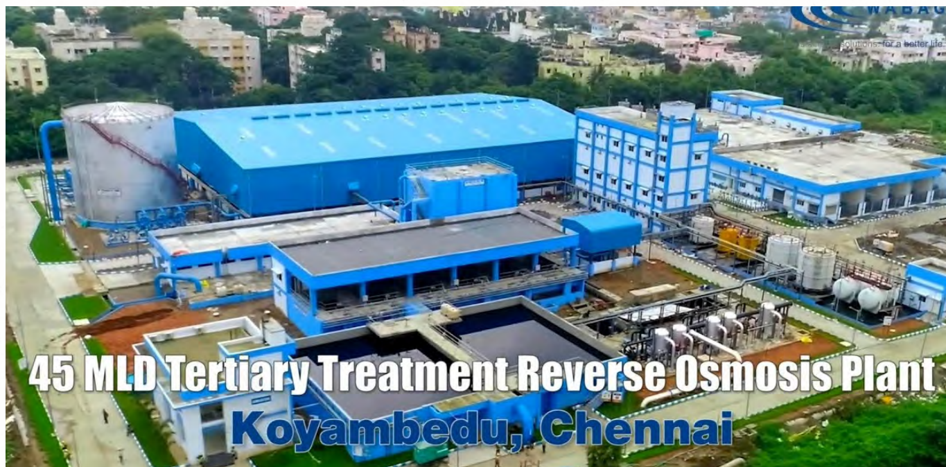
Figure 9.6: 45 MLD tertiary Treatment Reverse Osmosis Plant
